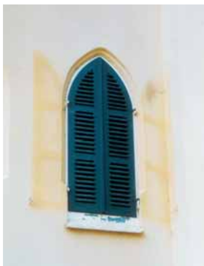
Colour changes around the shutters and under the eaves are clearly visible from the pictures.
