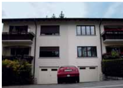
Soiling – practical example Private house in Lucerne, painted white at the same time. Left: silicone resin paint Right: silicate paint
