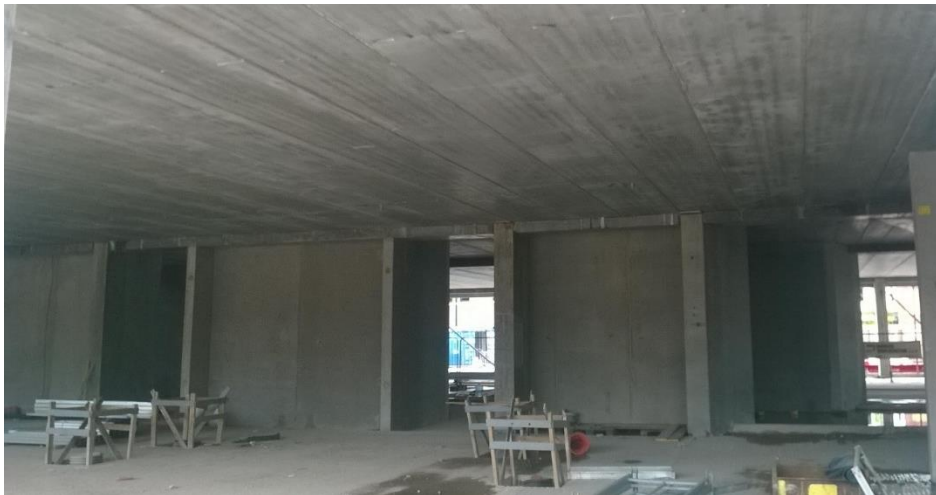
This photograph below shows the typical difference in a traditional (wall) and SCC (soffit) concrete finish
