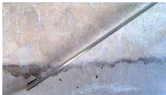
New concrete with defects that need to be refilled
