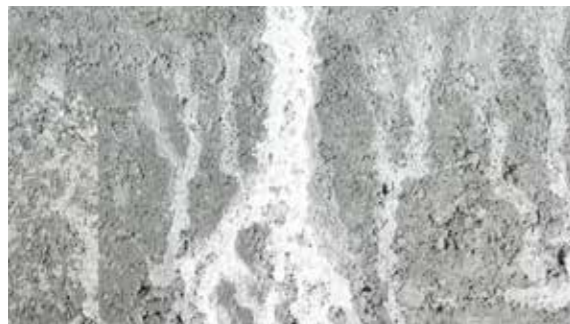
New concrete with severe blemishes
