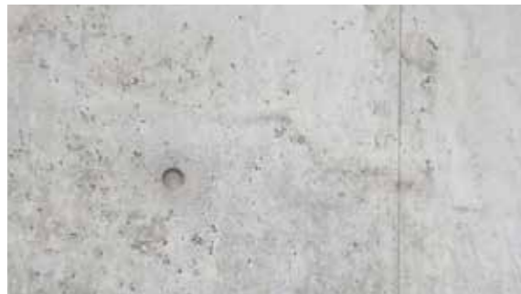
New concrete with slight blemishes
