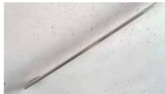
Refilled areas either strongly equalised or complete colour-matched mineral finish / © Arbeitsgemeinschaft Betonlasur
