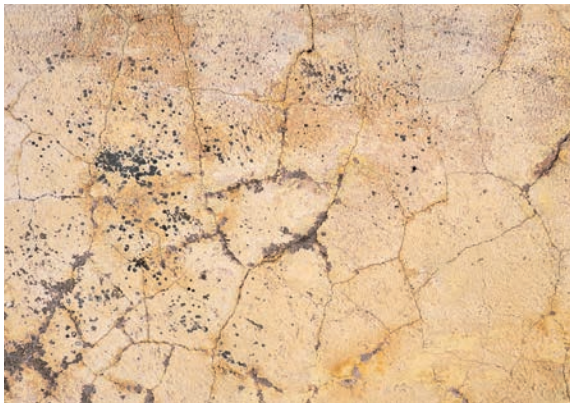
Cracked, old facade
